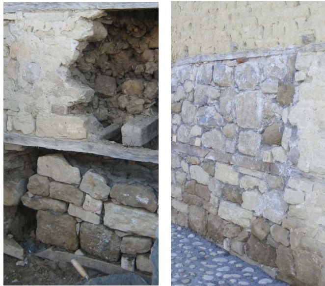
Figure 3.2 – Teknika prish-rinderto (foto IMK)
